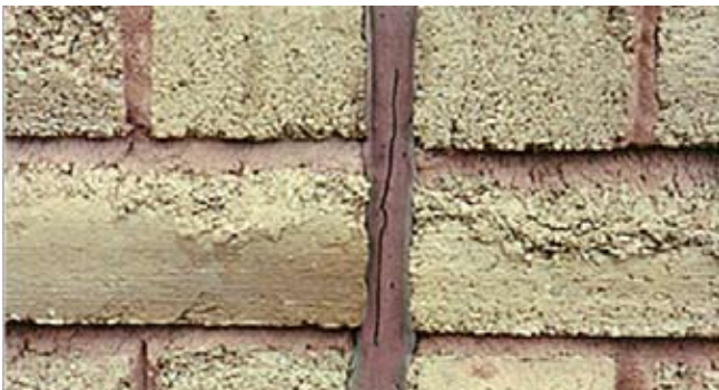
FIGURE 3.7 – SEALANT COHESIVE TEARING
