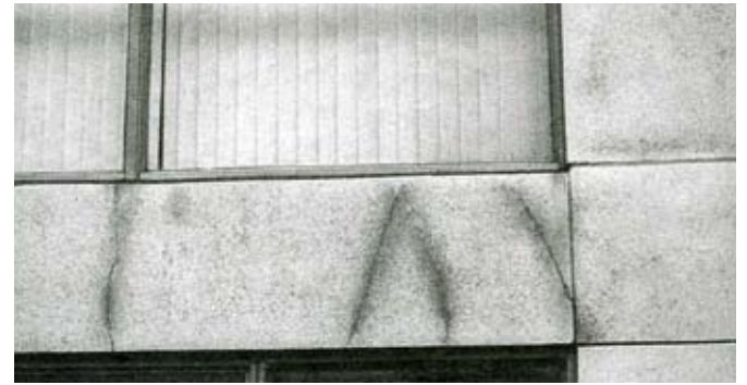
FIGURE 3.1 – WALL CRACKING PATTERNS
