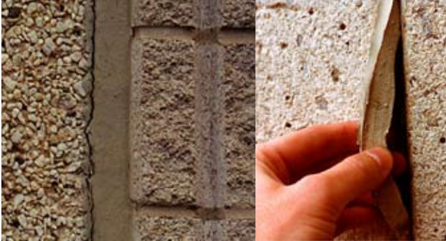
FIGURE 3.6 – SEALANT ADHESIVE BOND LOSS
